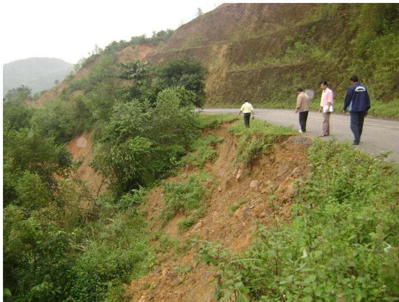
Figure 2-5: Fill slope failure
