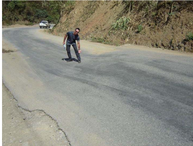
Figure 2-6: Failure through entire road bench on Road 13N
