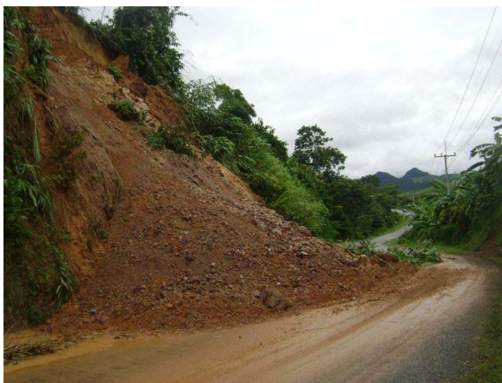
Figure 2-4: Failure of an over-steep cut slope
