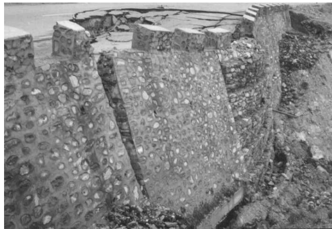
Figure 2-14: Failure following river flooding in front of wall 1
