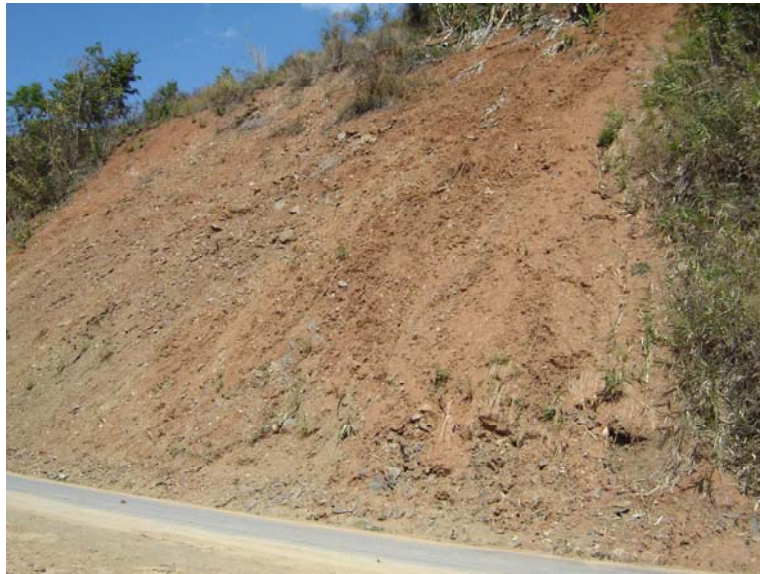
Figure 2-7: Typical slope erosion
