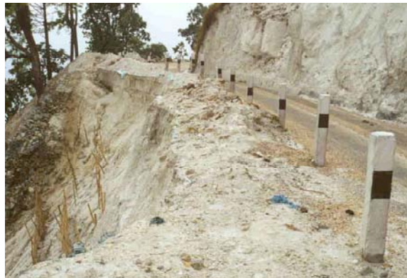
Figure 6-1: Failure below road protected by earth bund and marker posts
