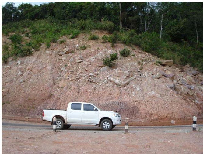
Figure 2-3: Shallow translational failure in colluvium
