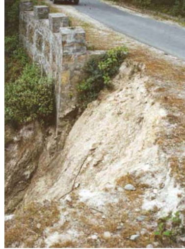
Figure 4-13: Erosion adjacent to wall
