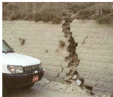
Figure 5-8: Cracking of masonry wall due to differential movement
