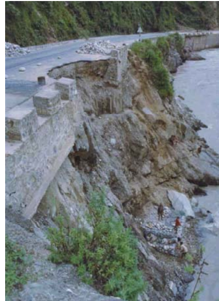
Figure 2-13: Masonry wall failure due to scour 1
