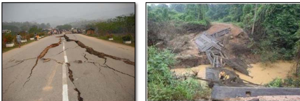
Figure 2.8: Road and bridge damage
