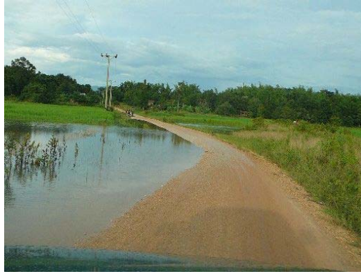
Flooding covering a rural road
