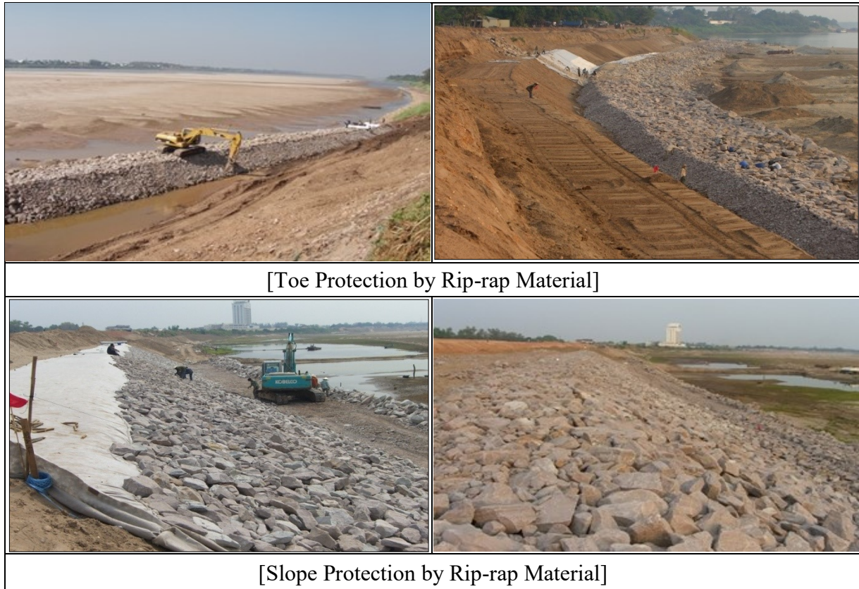
Figure A2-2 Case of the Rip-rap Protection in the MRIMP2, Vientiane Capital
